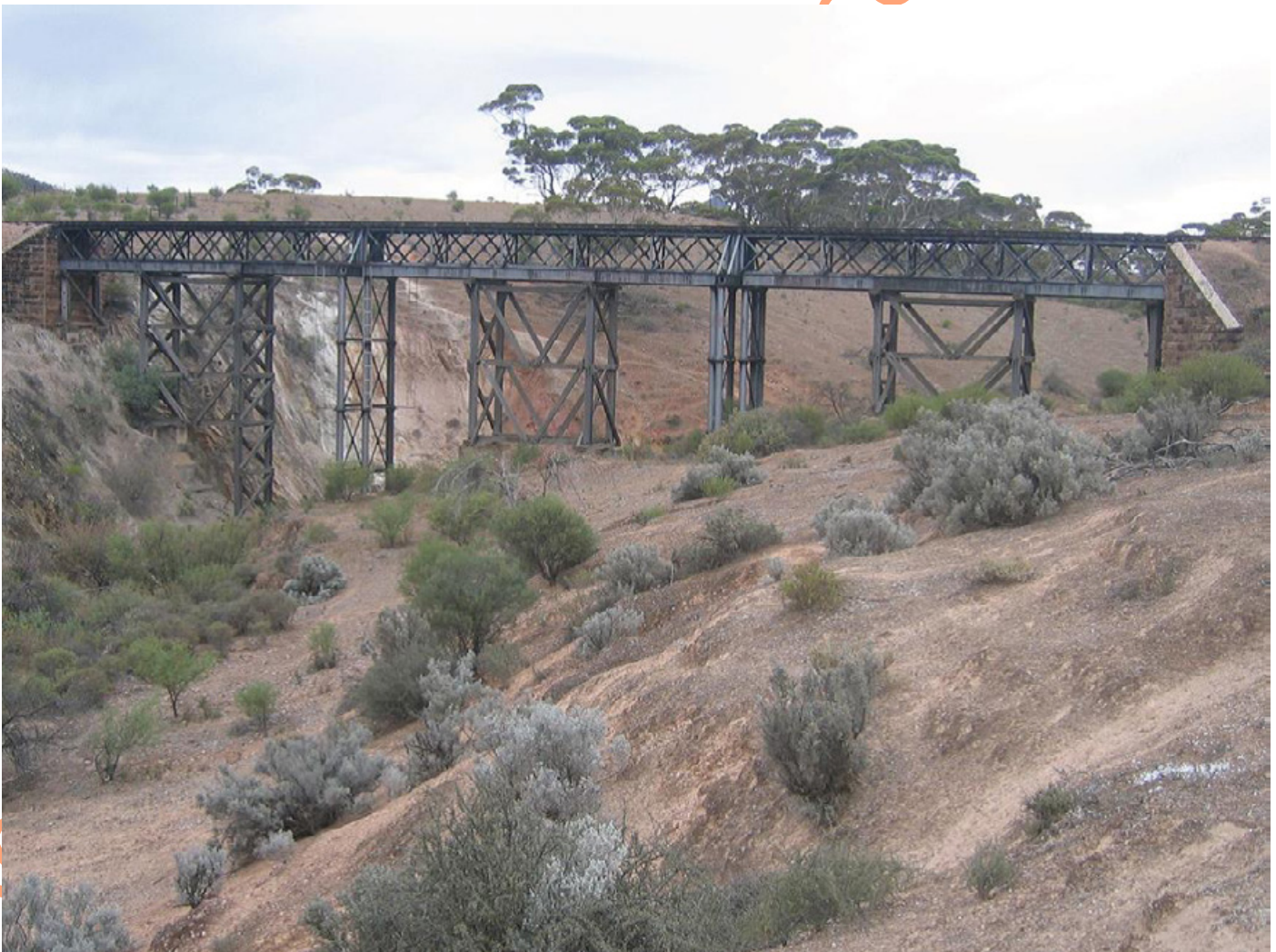
Lattice Bridge; Railway bridge and stone abutments. This is considered a good example of early railway infrastructure.
