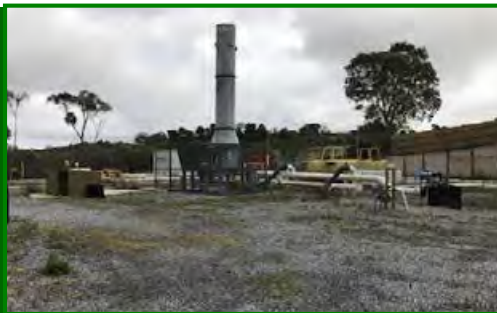
The LoCal flare Installed and operating at the Highbury landfill
