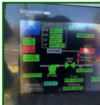
Control panel of flare operating
