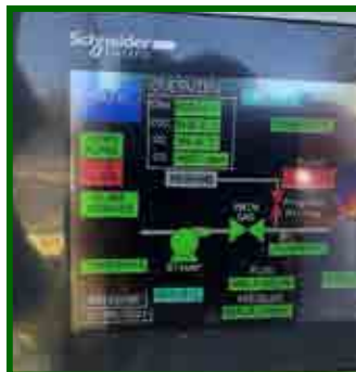
Control panel of flare operating
