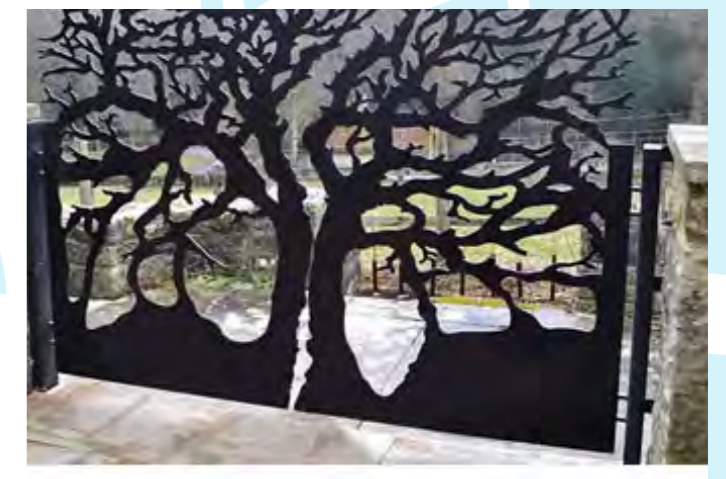
14 Unlocked permeable decorative gates to fire escape stair
