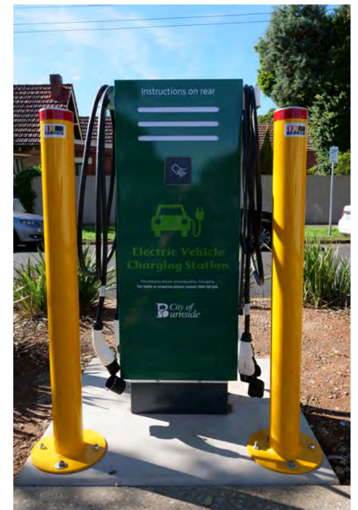
G Electric car charging stations
