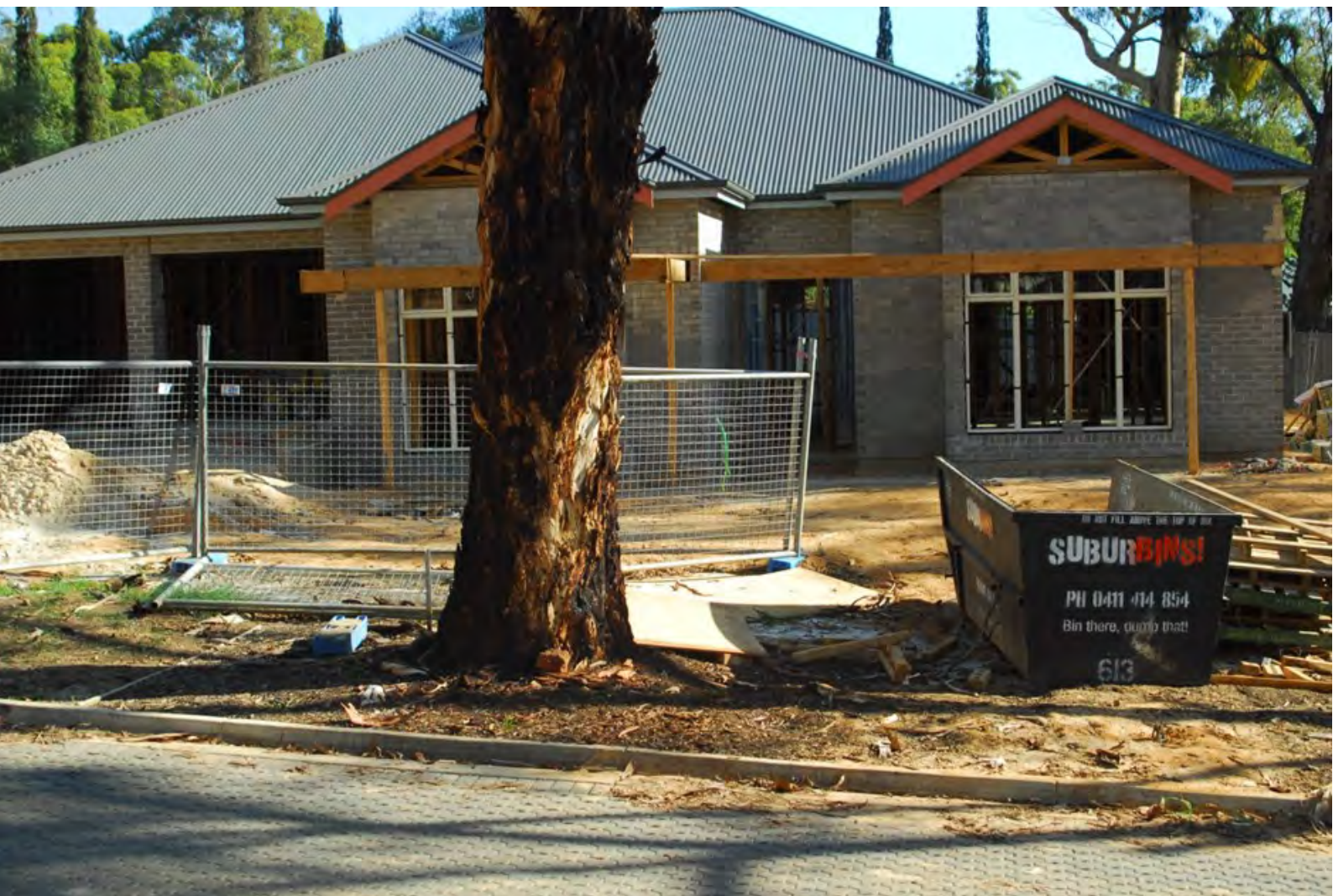
Photo: showing uncontrolled storage of building materials around a tree leading to soil compaction and trunk damage.
