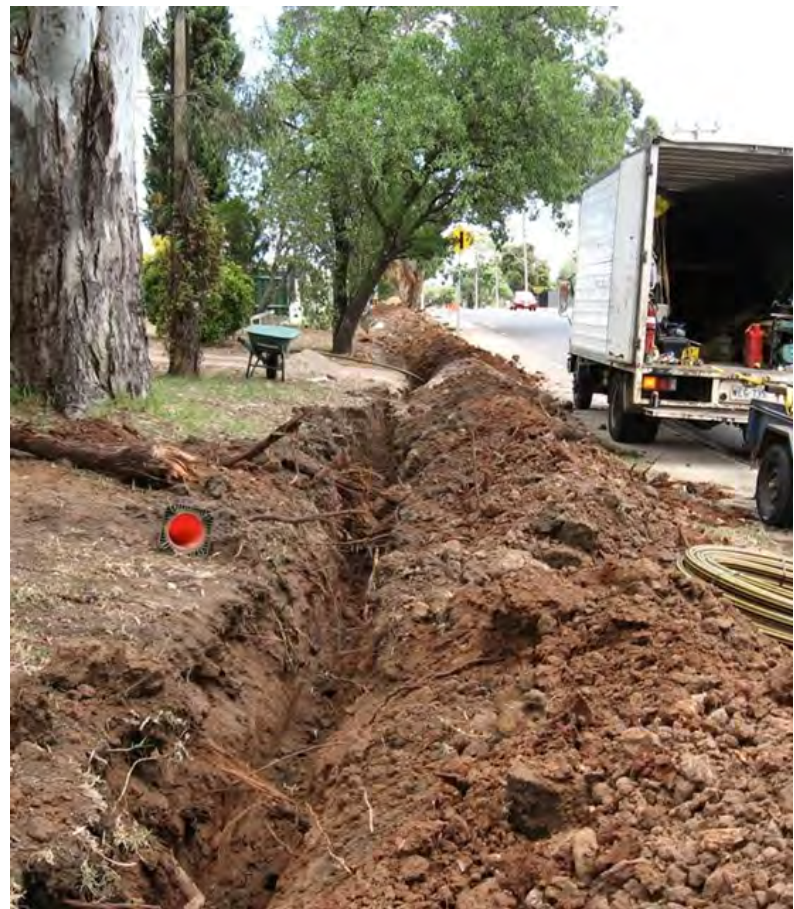
Photo: showing tree root damage from service trenching.
