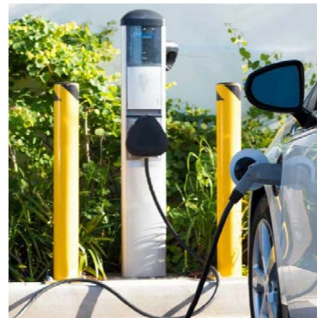
Electric vehicle charging stations
